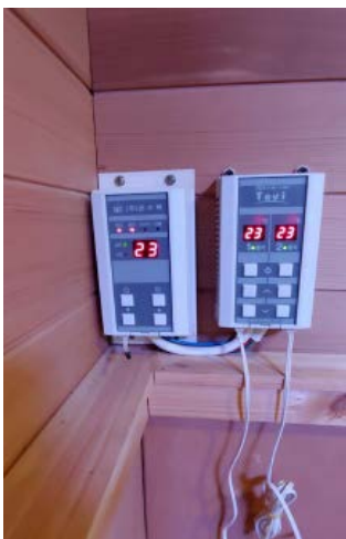
Figure 4. Temperature measurement inside simple office for small factories and temperature controller
